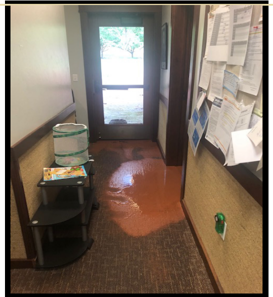
The staff entrance and server room where water and mud entered.
